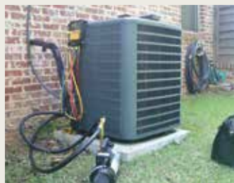
Pre-season HVAC tune ups
